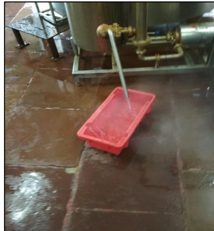
Figure 8: Condensate from hot water tank
