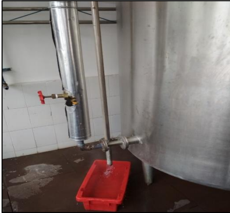
Figure 6: Condensate from CIP
